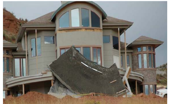
This collapse occurred during construction, not a fire. Three workers escaped injury by jumping out of the way at the last minute. The investigation revealed the contractor was using substandard materials and fasteners to attach the deck to the house.
