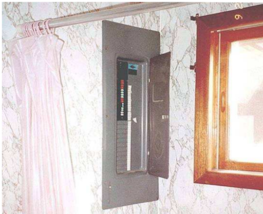
Breaker panel in the shower
