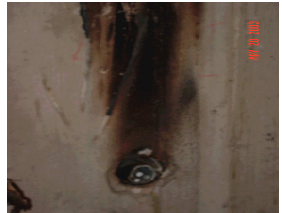
Breaker panel removed showing gas entry and burning through main electrical service feed
