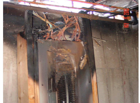
Breaker panel mounted on basement wall
